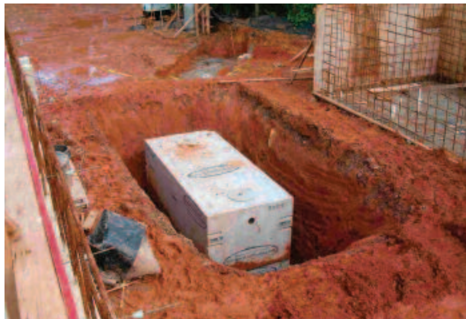
WATER CONTAMINATION? NOT WITH THE GREASE INTERCEPTOR IN PLACE. THE OWNER WAS INITIALLY CONCERNED WITH SEPARATING DOMESTIC POTABLE WATER CONTAINING CHEMICALS NOT FOR AVIAN CONSUMPTION – WATER QUALITY IN THE AREA WAS SUSPECT. KEEPING DOMESTIC WATER OUT OF THE PARROT'S REACH AVOIDED CONTAMINATION THREATS. CONSTRUCTION CREWS MANEUVER THROUGH THE CARIBBEAN NATIONAL FOREST IN THE HILLS OF PUERTO RICO.
